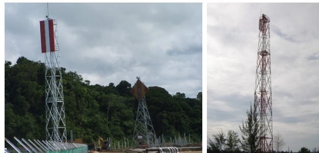
Construction of new leading lights and a 55m tower at Kuching port (left), and new leading lights and a 30m tower at Bintulu Port (right), both located in Sarawak.
